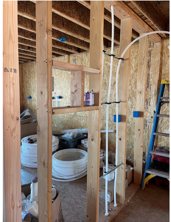
Plumbing lines installed in the mechanical room
