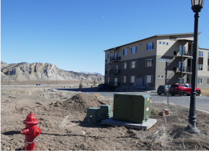
Newly Installed Transformer from Holy Cross Energy
